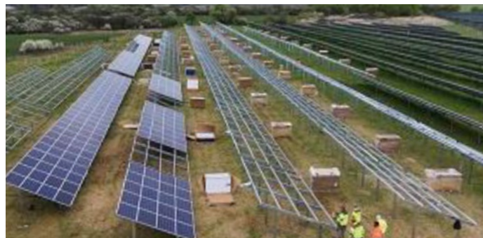
Digging of cable trenches and the relevant foundation work for the transformer stations.
