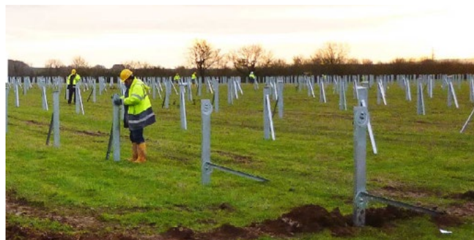
Ramming of the support profiles. Mounting of the project-specific substructure on the pole foundations.
